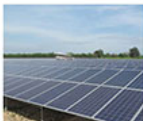
Solar Cell Supporting Structure
