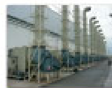
Bandai Wet Scrubber
