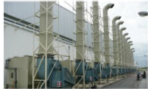
Bandai Wet Scrubber
