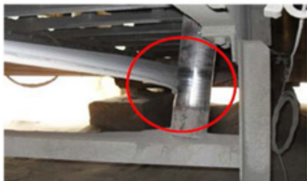
Misalignment at the return side
