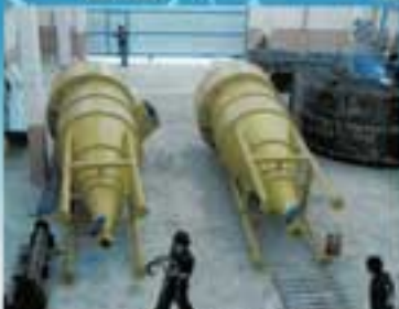
CYCLONE & ROTARY VALVE
