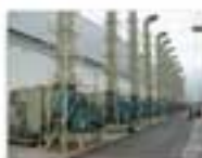
Bandai Wet Scrubber
